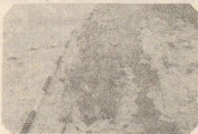
Photo 1. Damage of flexible pavement due to frost heave
