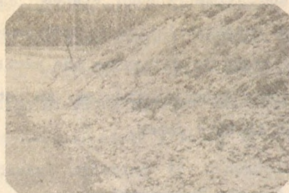
Photo. 3 Failure of the cut slope due to frost damage.
