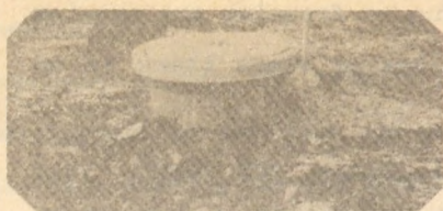
Photo 2. Uplift of manhole due to adfreezing force.
