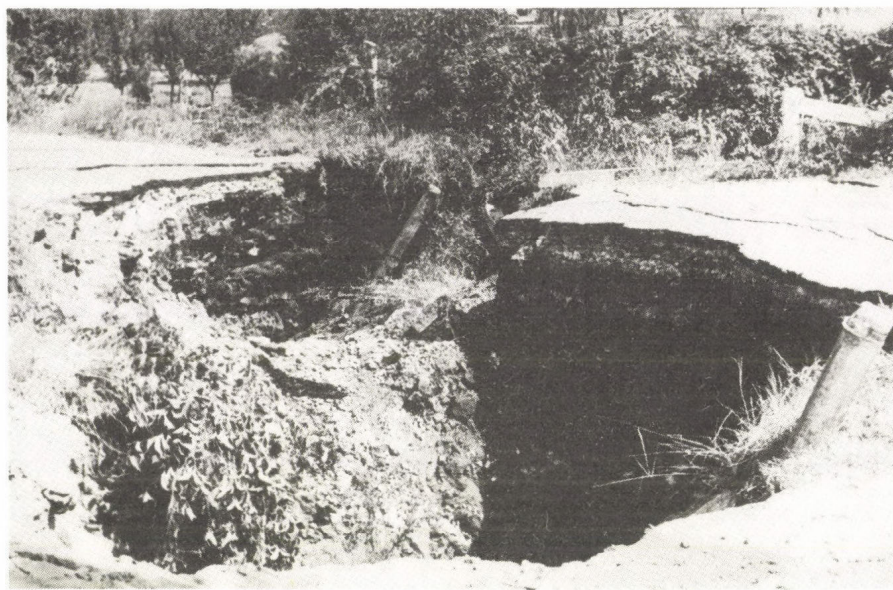
Picture 6. Collapse of an undermined road: Pécsbányatelep
