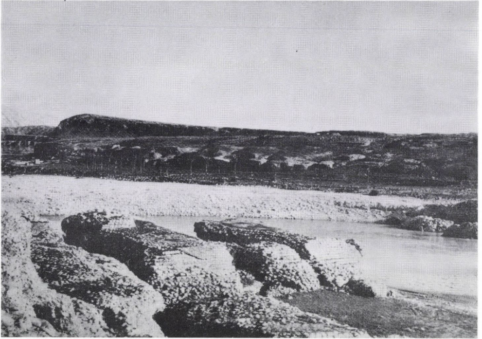
23. REMAINS OF BARRAGE BELOW PIERS OF ARRAJĀN BRIDGE, ON RIGHT BANK
